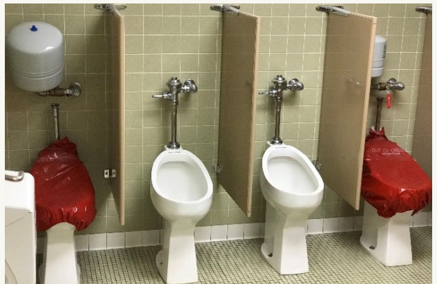
Restroom fixtures in need of replacement
