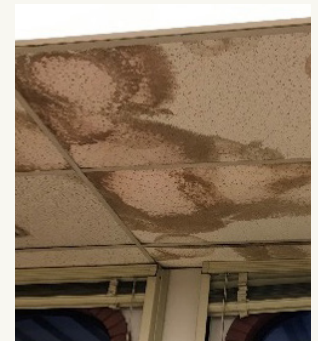
Leaking pipes have stained ceiling tiles
