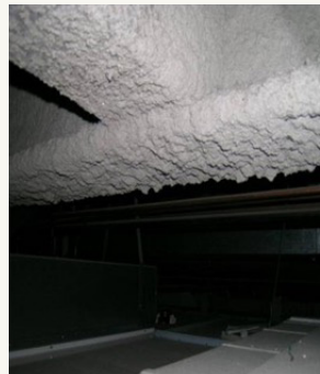
Spray-on asbestos over steel structure
